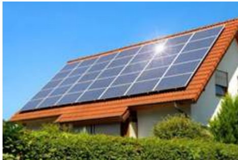
Gambar 10.15: PLTS Rooftop (bing.com/images-diakses 2024)
